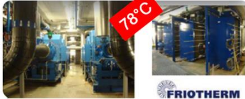
District heating & cooling (16.4MW)
